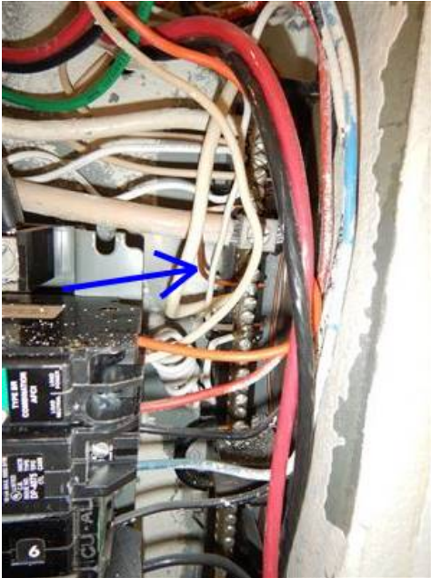
Photo 3-1 GROUND IN NEUTRAL BUS BAR
