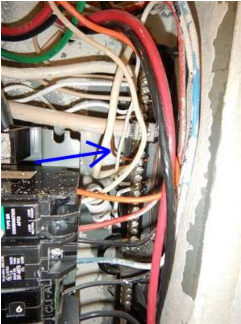
Photo 3-1 GROUND IN NEUTRAL BUS BAR
